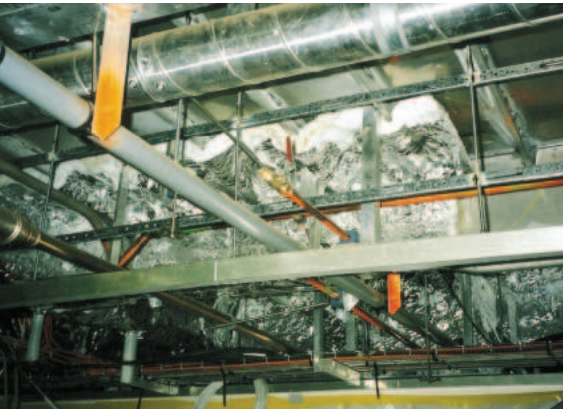
INSULATION IN THE ENGINE ROOM
